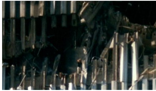
WTC-2 South Tower – No Raging Inferno
